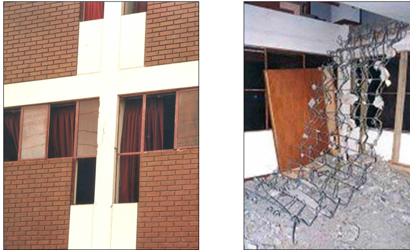
Fig. 3. “San Agustín” National University in Arequipa: short column typical failure (left), and library staircase collapse (right).
