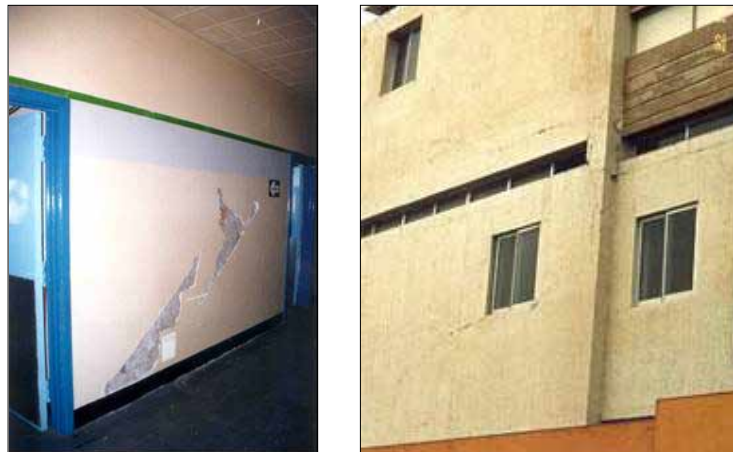
Fig. 6. Non-structural walls controlled lateral displacements and dissipated energy during the earthquake in hospitals: Arequipa (left) and Arica (right).
