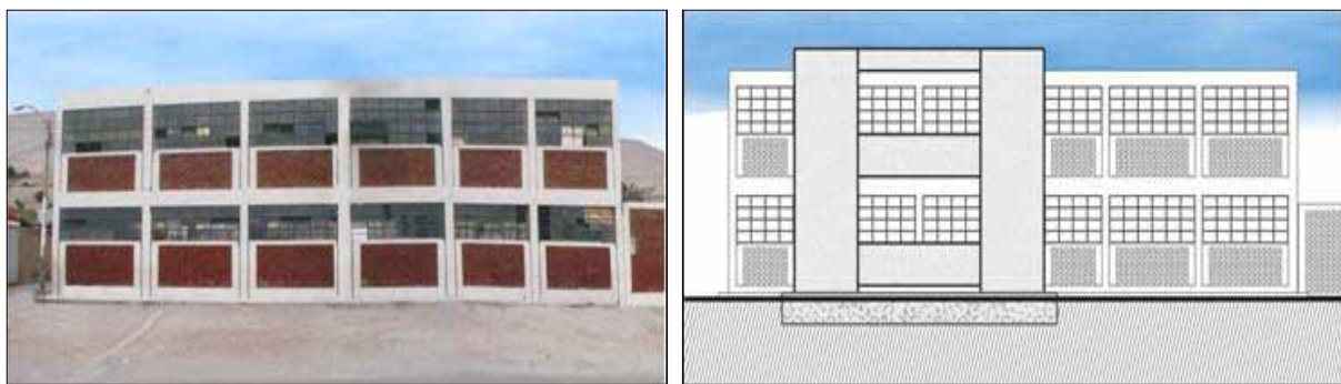
Fig. 9. Two-story school building damaged after the 2001 earthquake (left) and projected retrofitting in the longitudinal direction (right).
