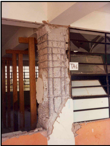
Figure 2. Short column failure, Nasca 1996 earthquake
