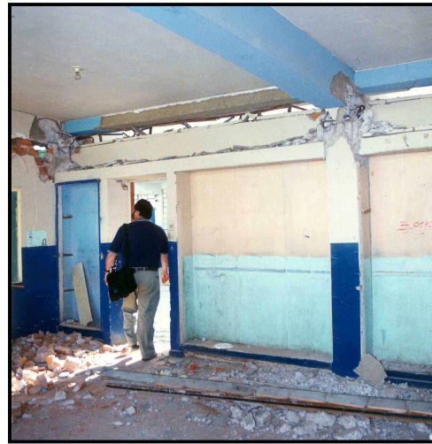
Figure 3. Generalized short column failure. Atico 2001 earthquake
