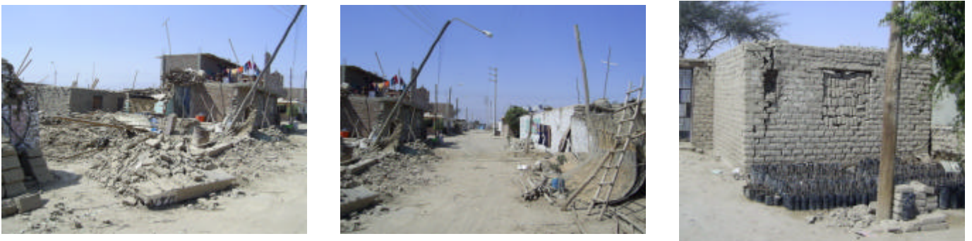
Figure 11. Traditional adobe houses with damage in Pachacutec
