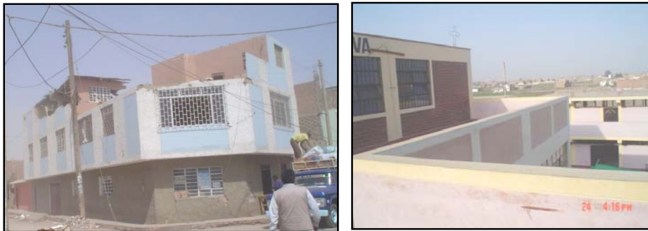
Figure 15. Parapet wall without bracing collapsed (left) and other adequately braced undamaged, both located on the third floor of their respective buildings, Pisco.
