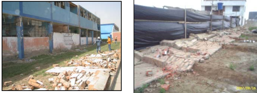
Figure 14. Perimeter walls collapsed by overturning. Masonry Piers are not enough.
