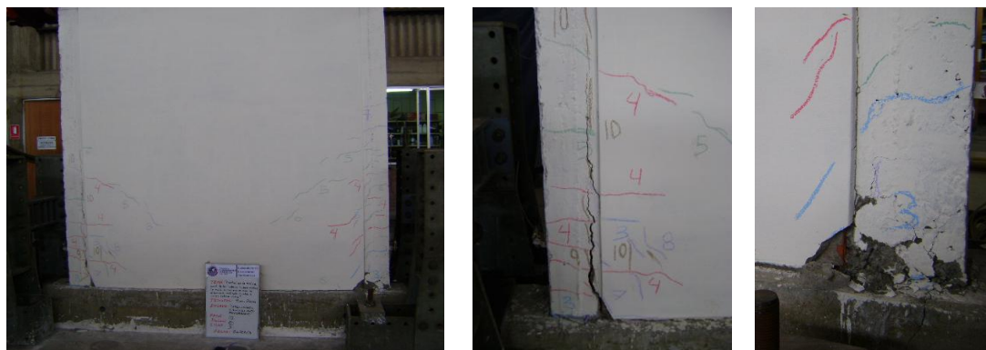
Figure 8. Wall W2 with detail of the column failures (bond and crushing)
