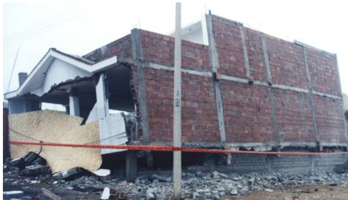
Figure 3. Collapsed house in the Atico earthquake.
