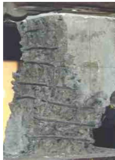
Figure 15. Concrete cover spalling and undamaged concrete core.
