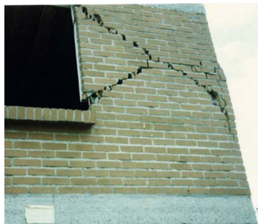
Figure 8. Shear failure due to wall stiffening.
