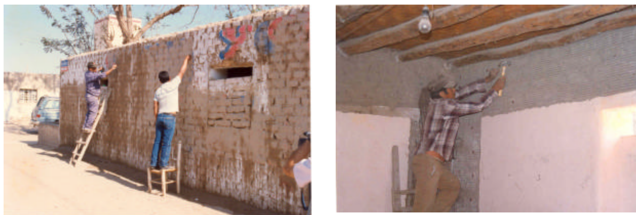
Figure 4. Adobe house in Guadalupe retrofitted in 1998 (left to right): marking horizontal strip at outside wall, nailing horizontal strip in inner side of wall.
