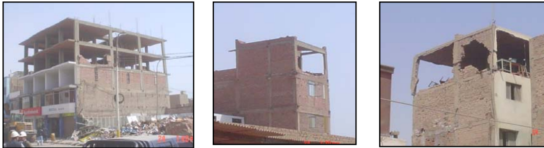
Figure 8. Overturning of masonry walls in high stories due to out-of-plane seismic forces.
