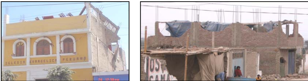
Figure 12. Collapse of roofs and walls in buildings without rigid diaphragm
