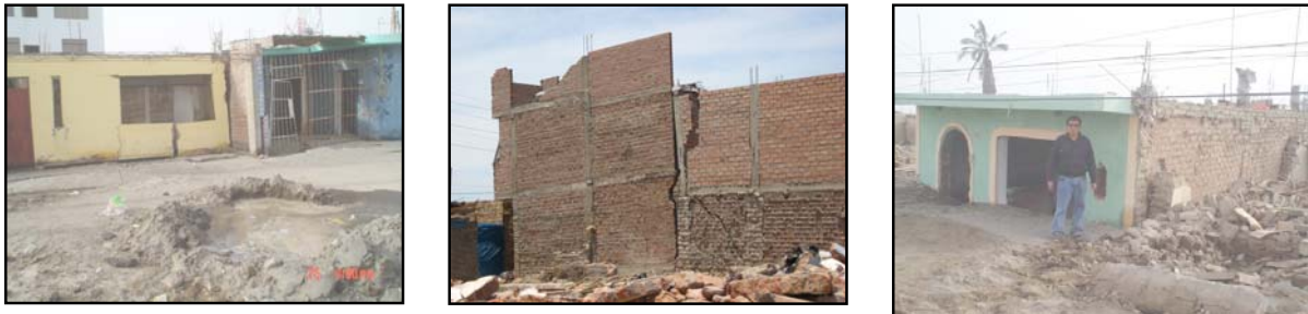
Figure 4. Affected masonry houses in Tambo de Mora.
