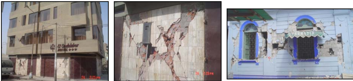
Figure 7. Inadequate masonry units used in Chincha, Pisco and Ica.
