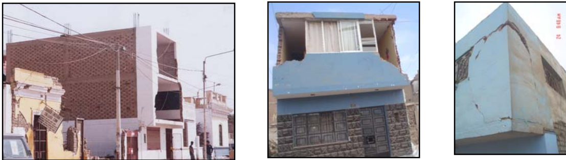
Figure 11. Failure of cantilever facades by out-of-plane forces
