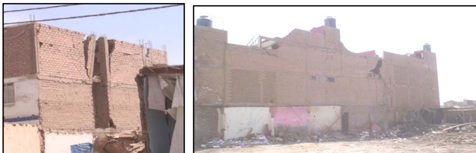
Figure 13. Walls without collar beam and column without continuity (left); bracing vertical columns too far apart each other (right); in both cases masonry failure is observed.
